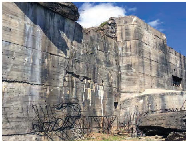
South wall of Watten, showing the successive layers of concrete poured beneath the jacked-up roof and twisted rebar where the control room was to be, LOx vents to right and severe bomb damage above. Photo Vincent Stenhouse
